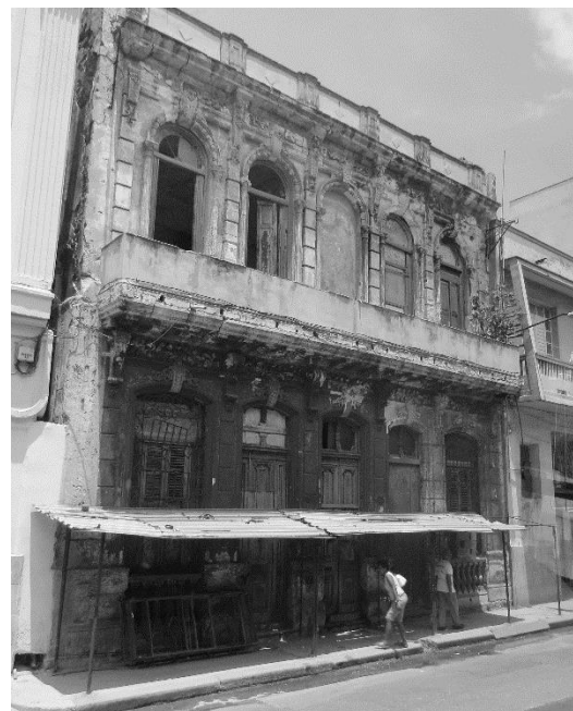
Deteriorated Apartment Building
