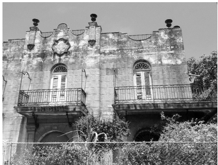
Partial View of Deteriorated Residence
