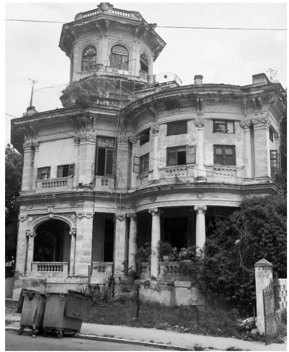
High Degree of Deterioration to Residential House
